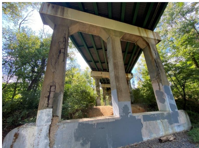
Figure 14 Exposed Substructure of One of the US 522 Bridges Vulnerable to Floodings Events
