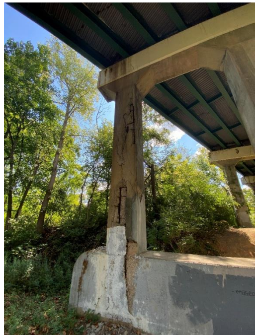
Figure 1 Deteriorated Column and Exposed Girders on One of the US 522 Bridges
