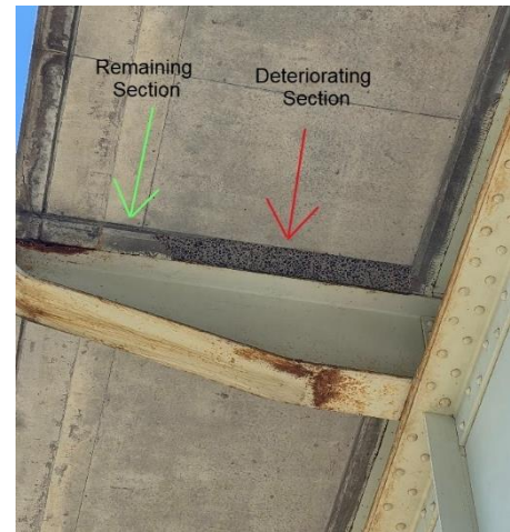
Figure 10 Deteriorating Underside of the Bridge with Falling Concrete Spalls That Pose a Safety Concern for Road Users on Limestone Road
