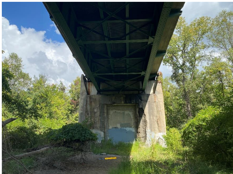
Figure 8 Deteriorated Columns under the Bridge Deck on One of the US 522 Bridges
