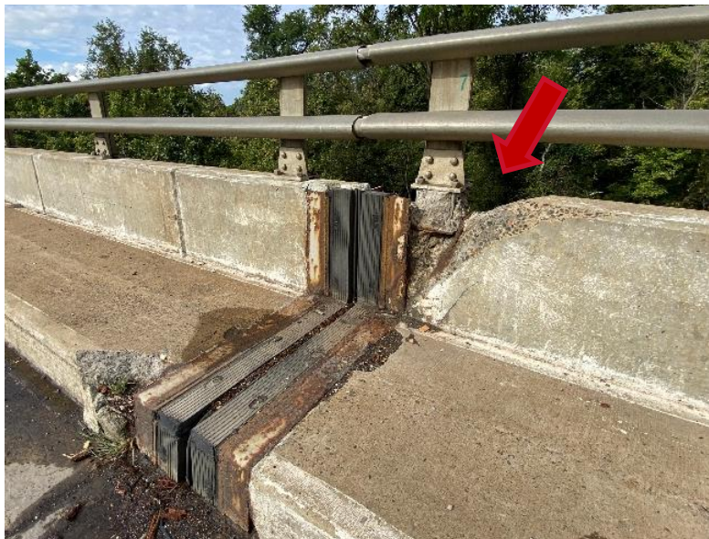
Figure 7 Broken Railing and Blocked Drainage on the US 522 Bridge
