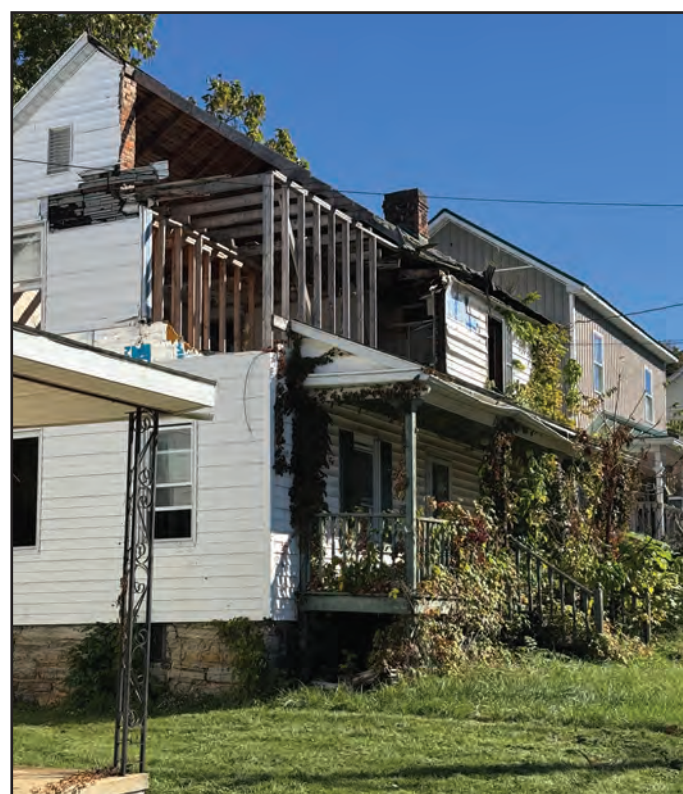
This downtown Hancock property designated as blighted raised questions about where things stand with plans to repair it.
