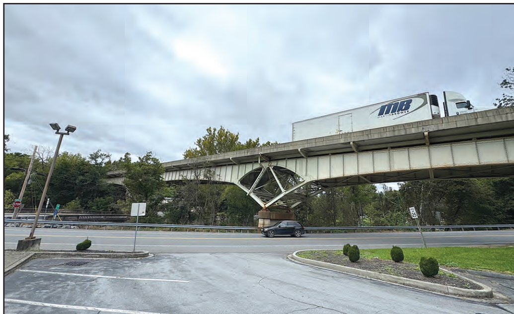
The U.S. 522 bridge in Hancock, shown on Monday, September 28, is on the list of “poor condition” bridges in the state of Maryland.
