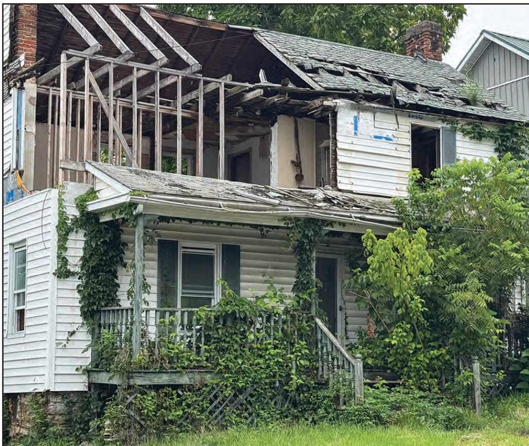
This High Street building is still the subject of negotiations between the town and owner on repairs or demolition. photo by Geoff Fox
