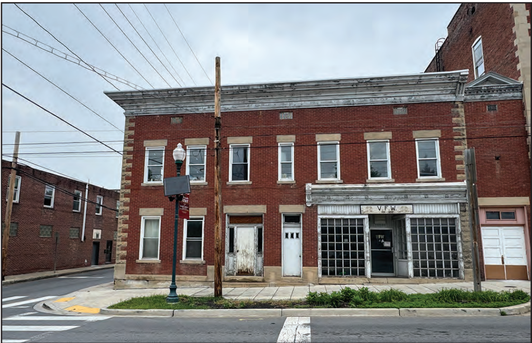
A Main Street building is still the subject of negotiations between the town and owner on needed repairs. photo by Geoff Fox
