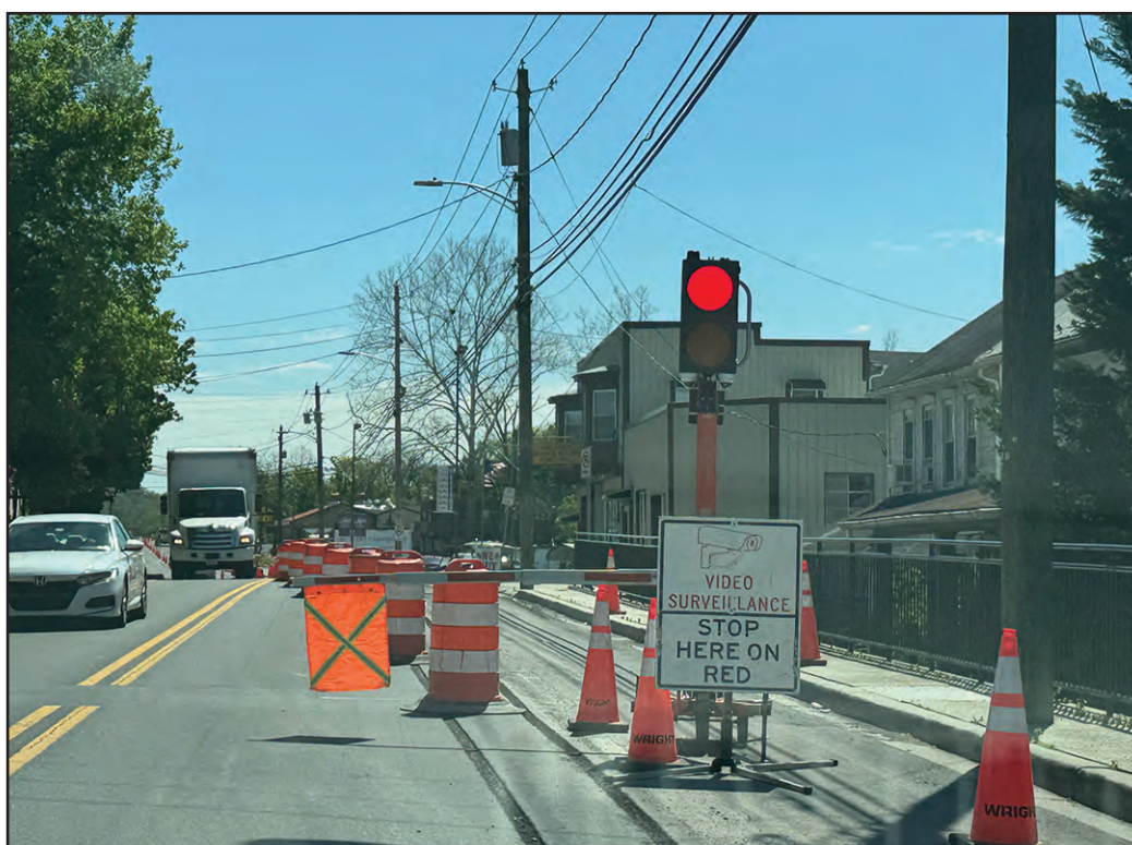
Columbia Gas of Maryland is laying new gas lines along Main Street in the area between 112 East Main and 170 East Main. To help with traffic control, they are using these red and yellow lights with flags.
