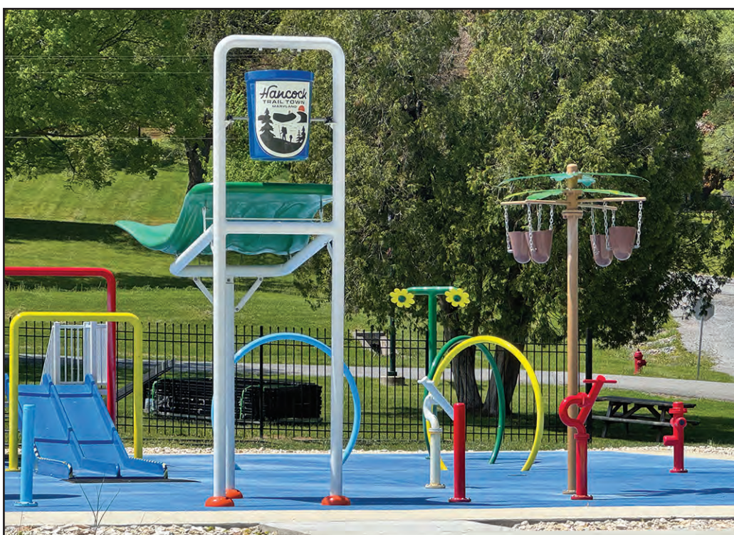
The town is installing a fence around the splash pad in Widmeyer Park before it opens later this month. The fence is to keep people off the splash pad when it is not open.
